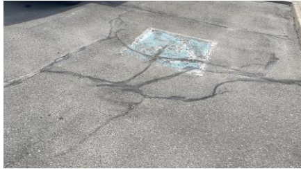
2000 In feet cracks
